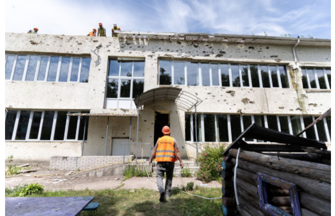
A kindergarten in Borodyanka in Kyiv Oblast under reconstruction thanks to support from Project HOPE. Photo by Nikita Hlazyrin for Project HOPE, 2023.
