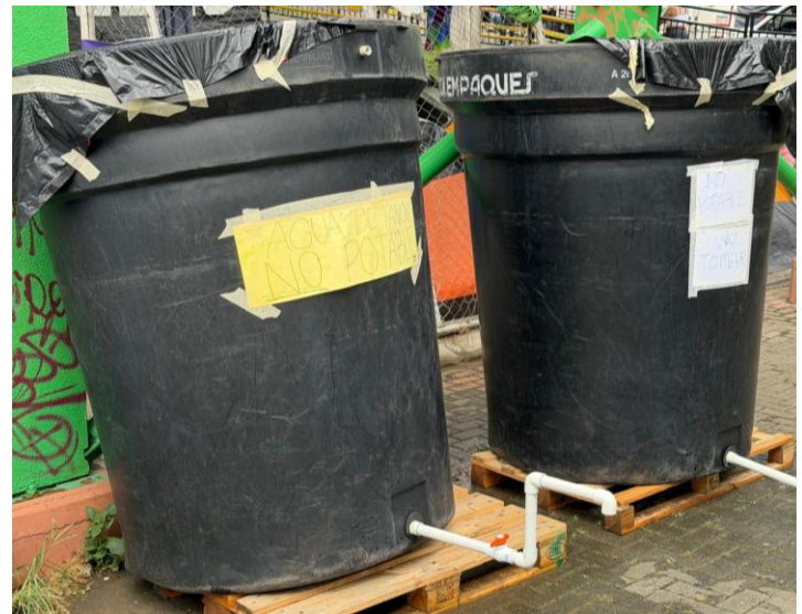
Water tanks (non-potable) in Polideportivo Mejia Robledo, one of seven shelters in Pereira. August 18, 2026
