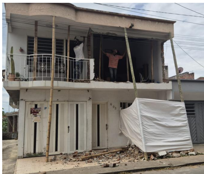
A damaged home is propped up with beams in Roldanillo. August 12, 2026
